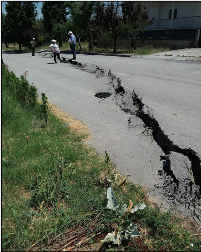
Fig. 12 Ground rupture at Anargyri village due to the landslide
