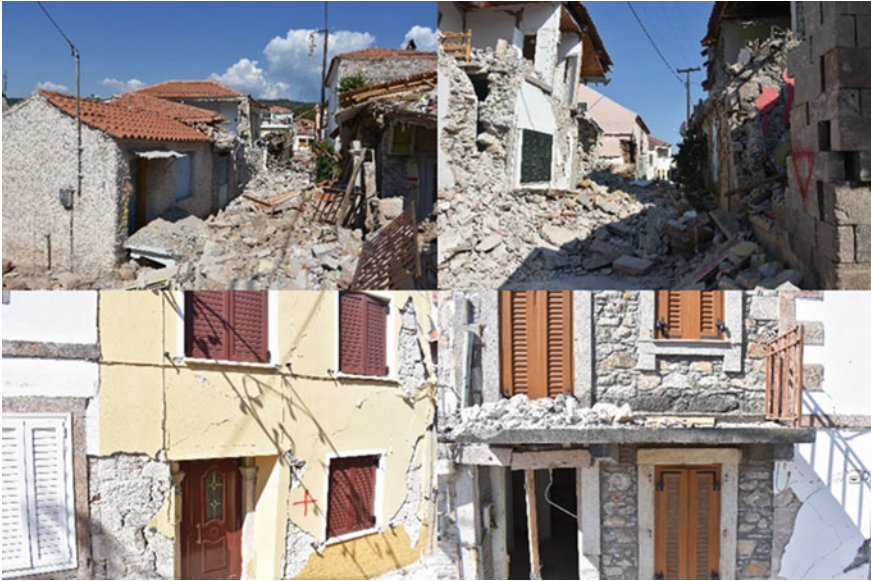
Fig. 4 Street conditions during surveys (up) and two damaged beyond repair buildings of the study area (down)
