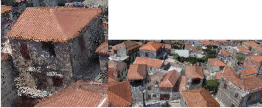
Fig. 10 Parts of the 3D point cloud derived by nadir and oblique images acquired on 25th June 2017, where building damages of grade 4 are clearly identifiable
