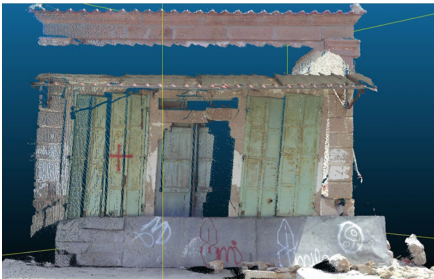
Fig. 17 An example from the third page of the proposed documentation of building damage assessment, which contains the 3D point cloud derived by TLS. The 3D measuring tool permits the accurate measurement of distances, angles and volumes
