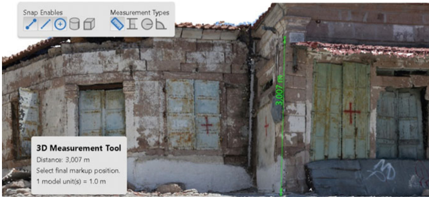
Fig. 16 An example from the second page of the proposed documentation of building damage assessment which contains the 3D point cloud obtained by the high-resolution terrestrial photos. The 3D measuring tool permits the accurate measurement of distances, angles and volumes
