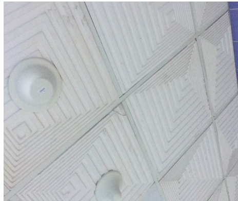
Fig. 3. DASs installed in the ceiling of the building indoors connected to the splitter.
