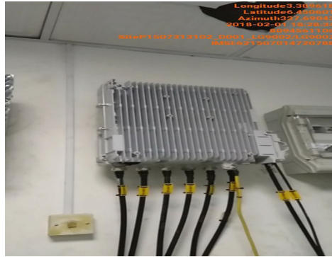
Fig. 2. Splitter connected to DASs and NodeB site on Tower Roof using coax cable.
