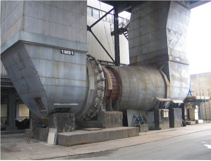
Fig. 1. Flue gas duct with an axial exhaust fan
