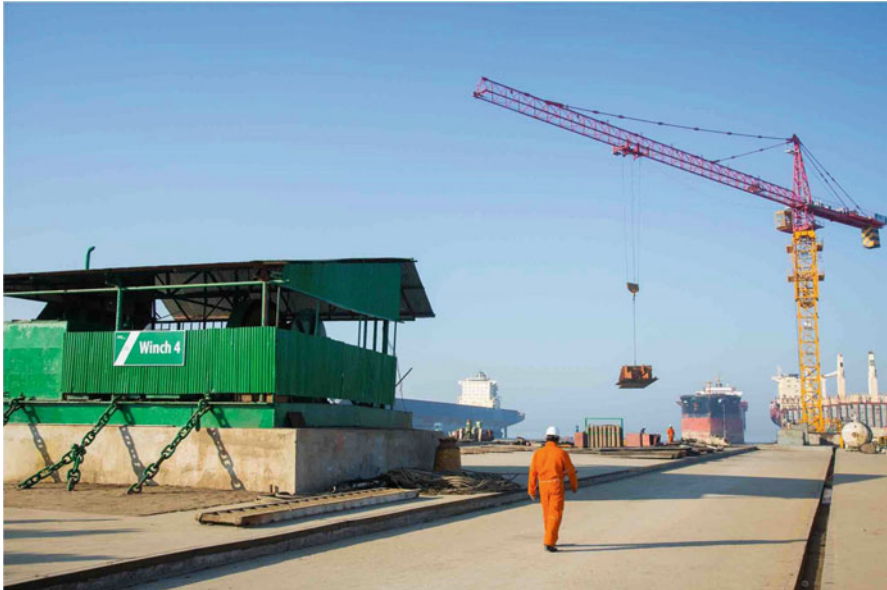
Fig. 6.16 PHP Shipbreaking and Recycling Industries Ltd. in Chittagong Bangladesh with HKC SOC by RINa
