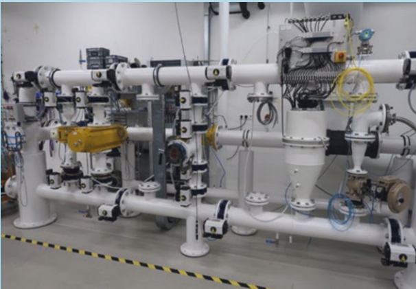
↑ One of VSL's gas flow calibration facilities, showing various reference standards against which other flow meters can be calibrated. (courtesy of VSL / photo by Fons Alkemade)
