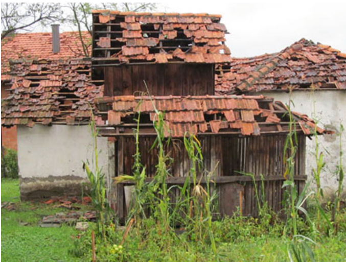
Fig. 17 South Brčko District—Damage to immovable property caused by the hailstorm on June 25, 2014
