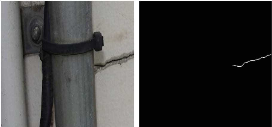
Fig. 6. Automatic crack detection in an image of a scene in building. Left image is the input crack image, right image is the detected binary crack map
