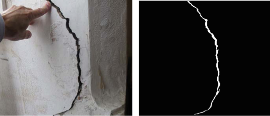
Fig. 4. Automatic crack detection in a concrete column. Left image is the input crack image, right image is the detected binary crack map
