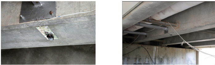
Fig. 12. SHM installed as scalable package 3 (ACM)
