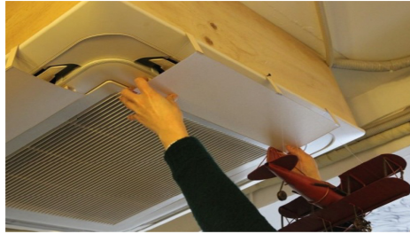
Fig. 8. Wind guide plate to divert cold wind from air conditioner to other direction
