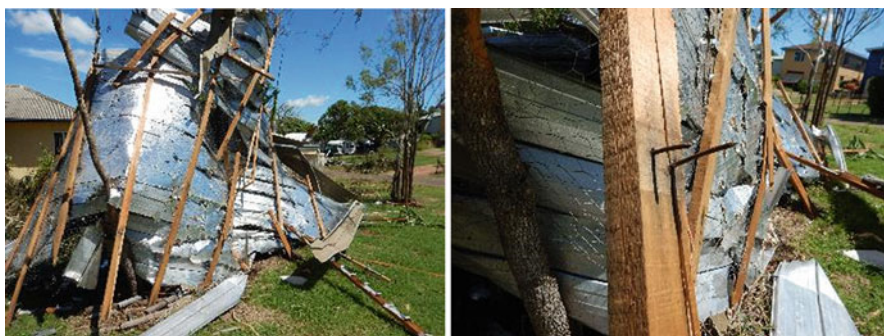
Fig. 10.5 Wind-induced failure of a metal cladding roof (left) at the batten to rafter connection (right) during Cyclone Marcia (2015) in Yeppoon, Australia
