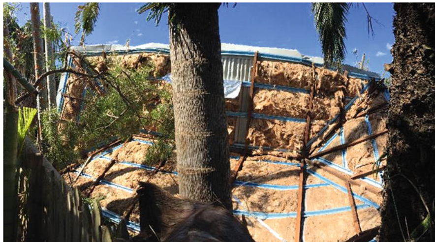
Fig. 10.4 Wind-induced failure of a new (<1 year) metal cladding roof on an old house at the rafter to top-plate connection during Cyclone Marcia (2015) in Yeppoon, Australia – there appeared to be no retrofitting of the weaker connections
