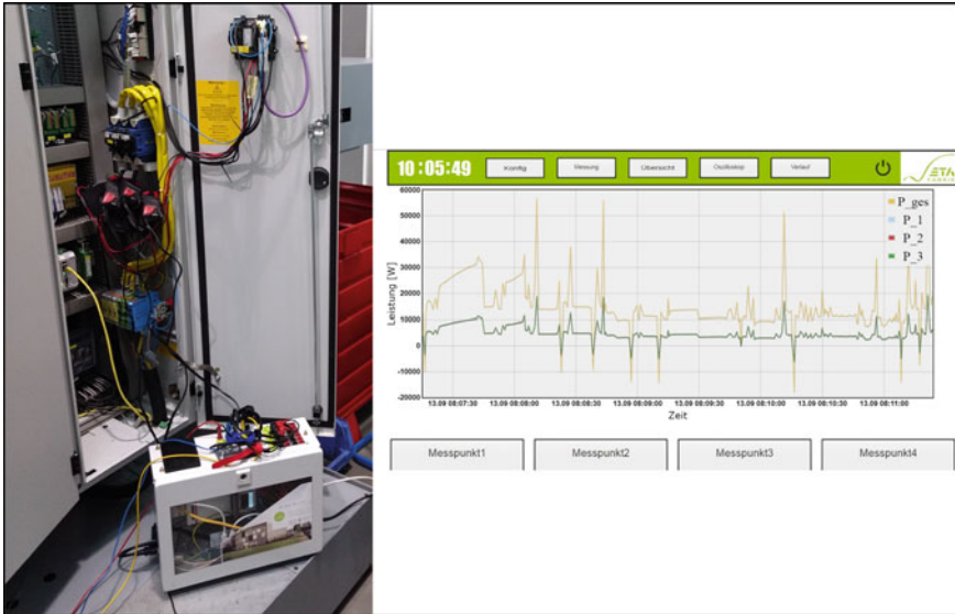
Fig. 5.8 Electric Power Measurement with mobile measurements device on the EMAG VLC 100Y turning machine
