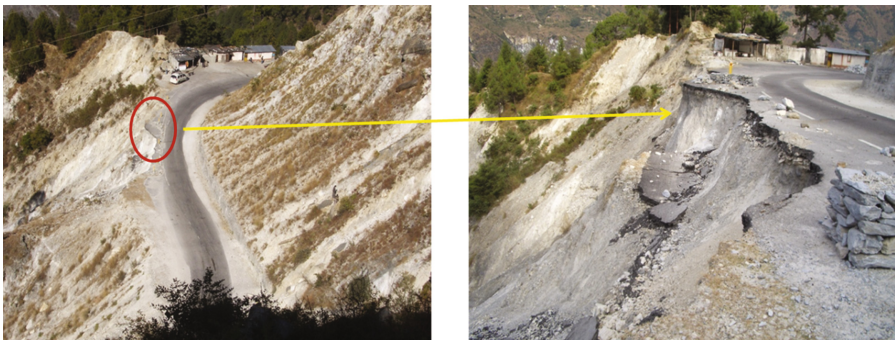
Fig. 3. Highway at risk due to debris slide
