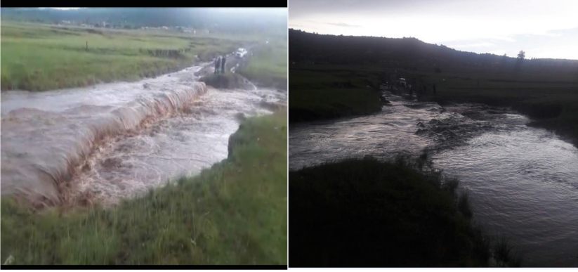
Fig. 2. Low bridges over flowing water due to heavy rain in Eastern Cape, South Africa (Taken by authors).
