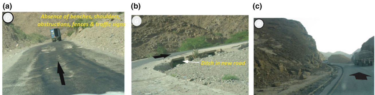
Plate 3 a The absences of benches, shoulders, obstructions, fences and traffic signs; b Ditch in the new road, c Dangerous curvatures of the new road
