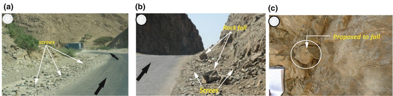
Plate 1 Different types of rock falls along Alagaba new road. a Debris flow; b Rock falls
