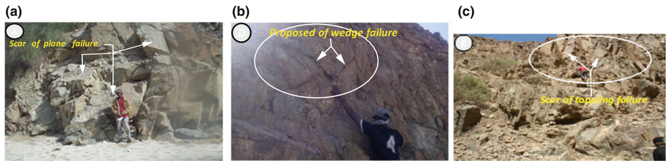
Plate 2 Different types of slope failures along Alagaba new road. a Plane failure; b Wedge failure; c Toppling failure
