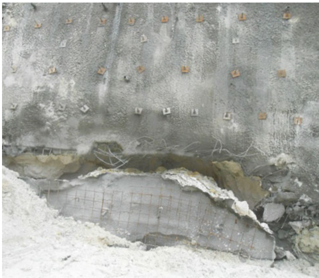
Fig. 4 Collapses occurred below the installed support measures
