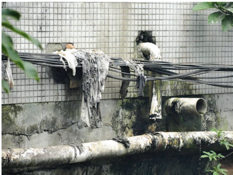
Fig. 12 Further unclear situation of undesired wastewater discharges
