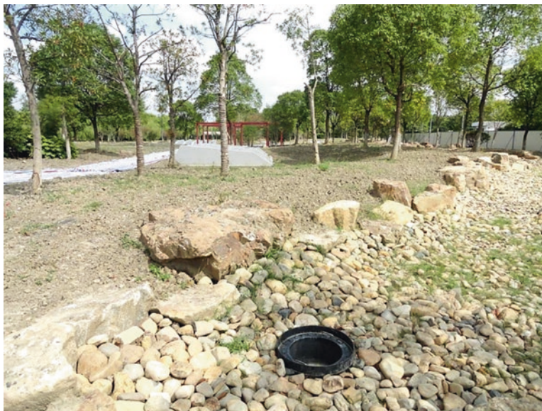
Fig. 5 Rain garden under construction in the first round Sponge City Jiaxing (September 2016)
