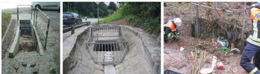
Fig. 13 Stormwater inlets with three-dimensional screens to avoid blocking
