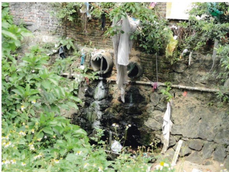
Fig. 11 Unclear situation with regard to undesired wastewater discharges
