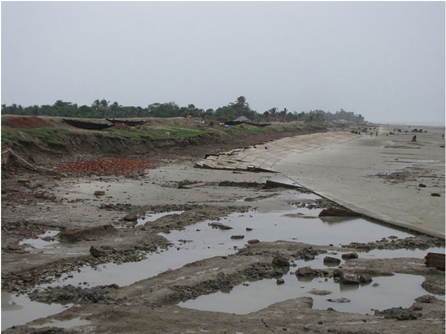
Erosion and embankment collapse (Courtesy A. A. Danda)
