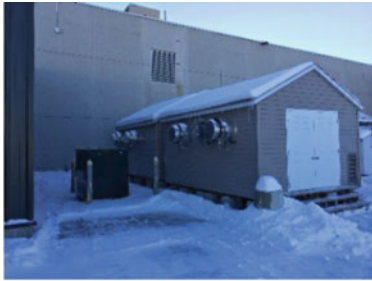
(a) Test Bench Exhaust Fans
