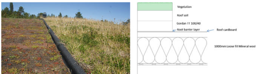
Fig. 1 Left: picture of the green roof in Kiruna with sedum on the left and sedum wild flowers and grass on the right. Right: schematic picture of the roof sections
