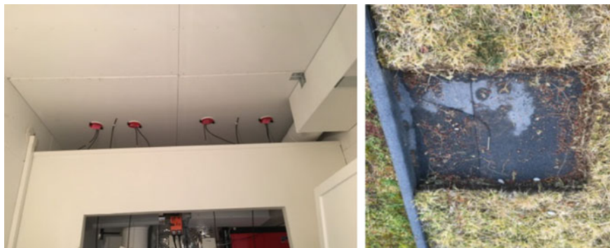
Fig. 2 Left: installation of the heat flux sensor pairs and the thermocouple. Right: removed part as reference area
