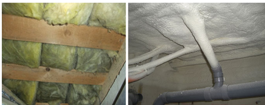
Fig. 2 Wall insulation (left: before renovation) and undersurface of the floor (right: after renovation)
