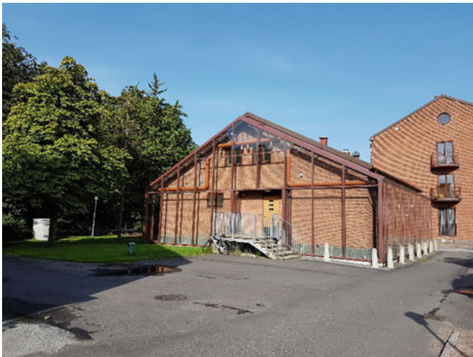
Fig. 1 The studied building located in Sege Park in Malmö, with the added glazing visible on the south and east façade. The inlet pipe to the added concrete duct for the cooling of the cavity can be seen on the left part of the picture
