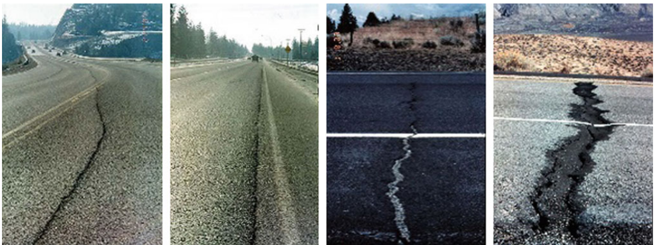
Fig. 66.3 Top two retrieved images using the “longitudinal crack” and “transverse crack” keywords (further annotated with “non-fatigue crack”)
