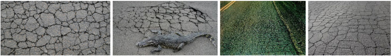
Fig. 66.4 Top two retrieved images using the “alligator crack” and “fatigue crack” keywords (further annotated with “fatigue crack”)
