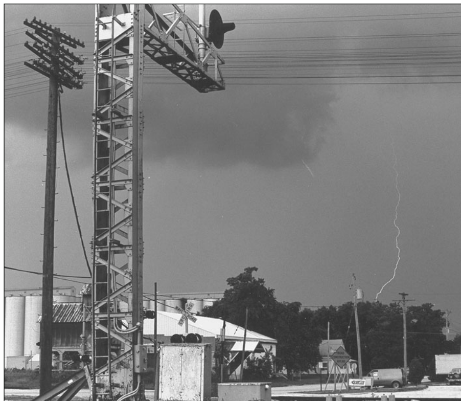
Fig. 2.17. Electrical storms also cause problems. Lightning strikes can cause power outages and loss of communications. Here a lightning strike hits just west of a Wabash signal bridge.
