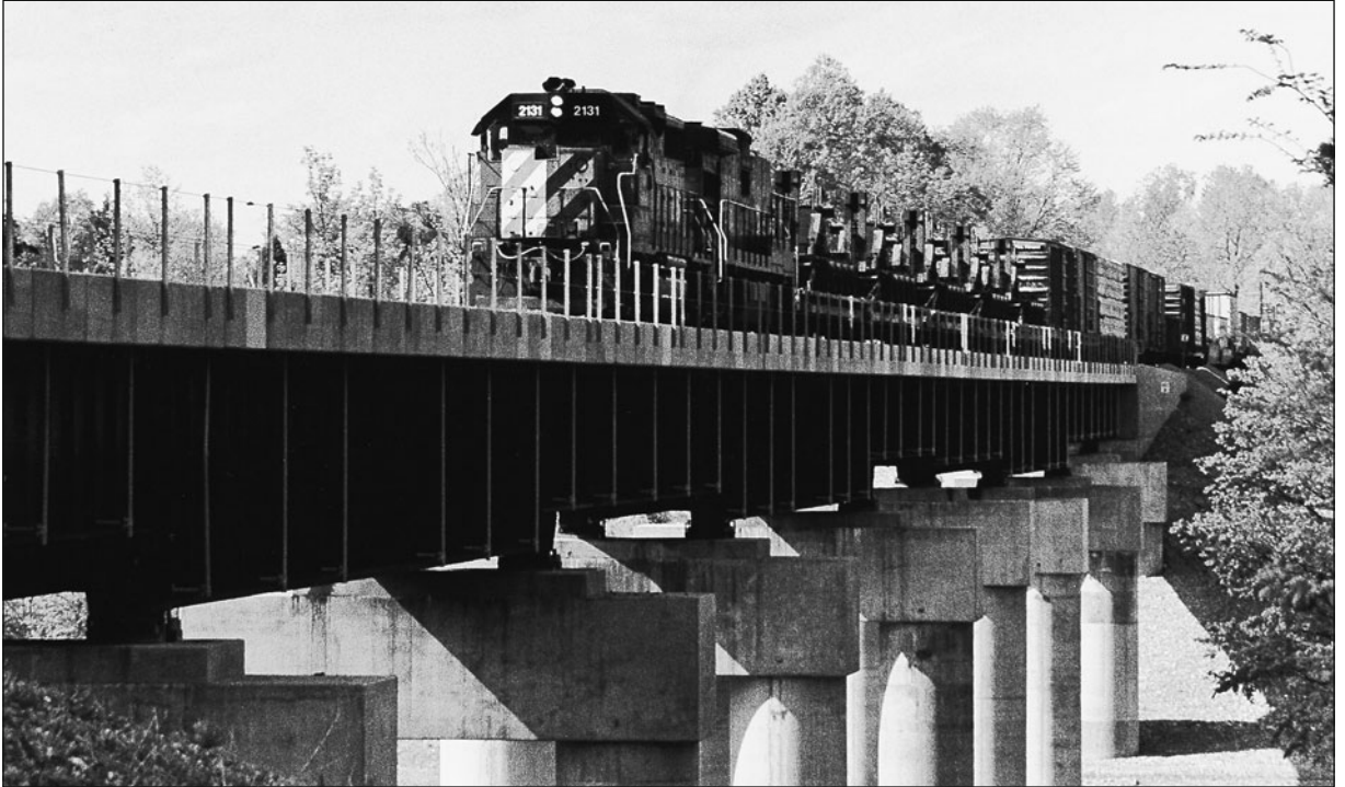
Fig. 5.3. Floods create the need for costly new bridges. The UP built this viaduct-style trestle across a creek valley in 1990 to replace an aging steel trestle.
