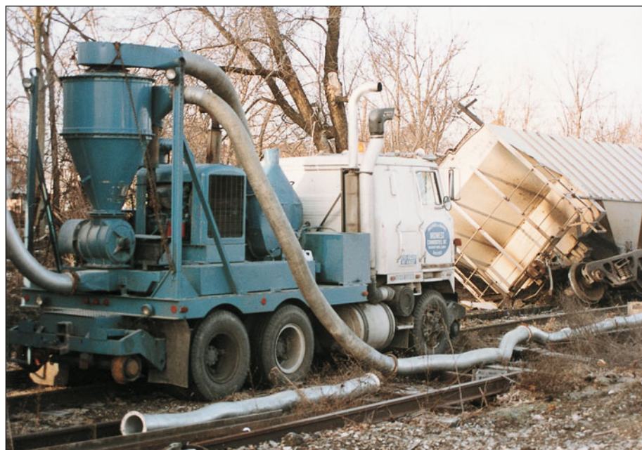
Fig. 5.20. A wrecked grain train has spilled corn everywhere, and this special truck can literally “vacuum” spilled grain from along the track and from inside wrecked cars.
