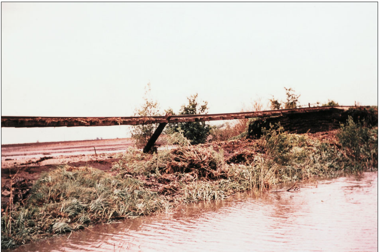
Fig. 3.17. One of the many washouts from the extensive snowmelt flooding in California in late December 1996.
