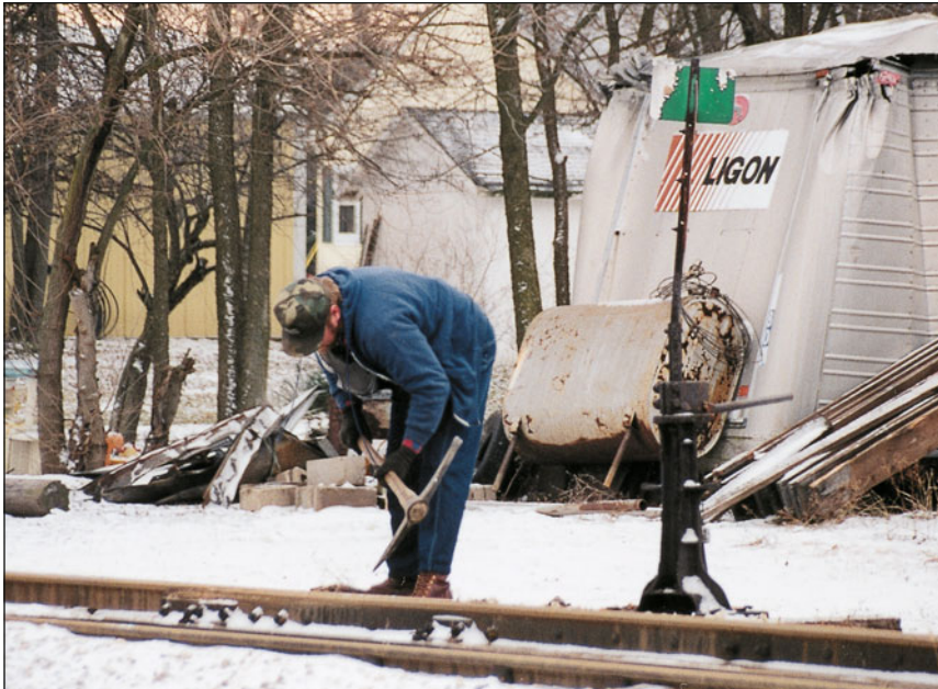
Fig. 4.11. A workman uses a pick to dig the snow and ice from a frozen switch.
