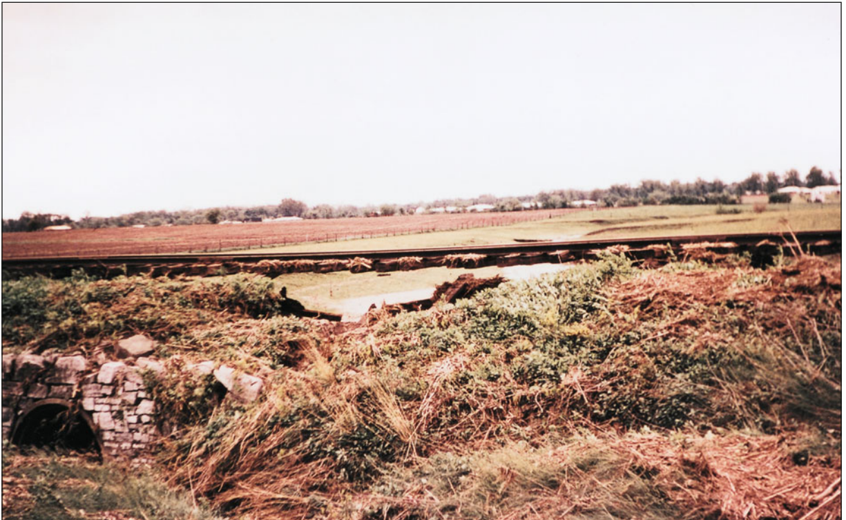
Fig. 2.20. Flooding leads to washouts of roadbeds like this one in Arkansas. The major activity in the following days involved restoring the earthen fill and rebuilding the small bridge (left) that was enlarged to better handle future high waters.
