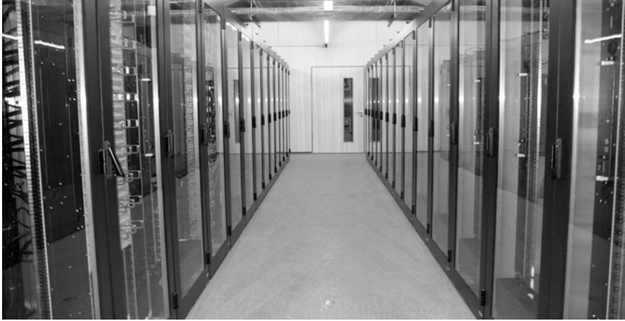
Fig. 6.62 A modern server room in a computing center of a university hospital
