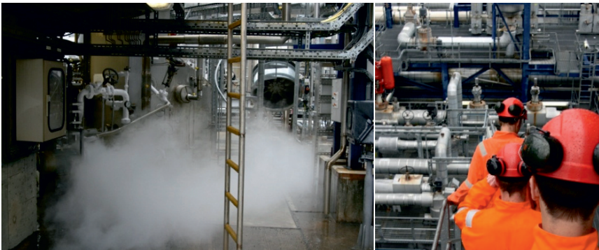
Figure 2. A typical oil and gas plant environment.
