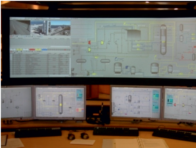
Figure 3. A control station.
