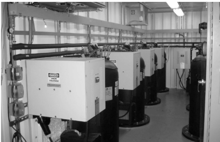
Figure 9.15. The view of Beacon Power's Smart Energy Matrix™ [17]
