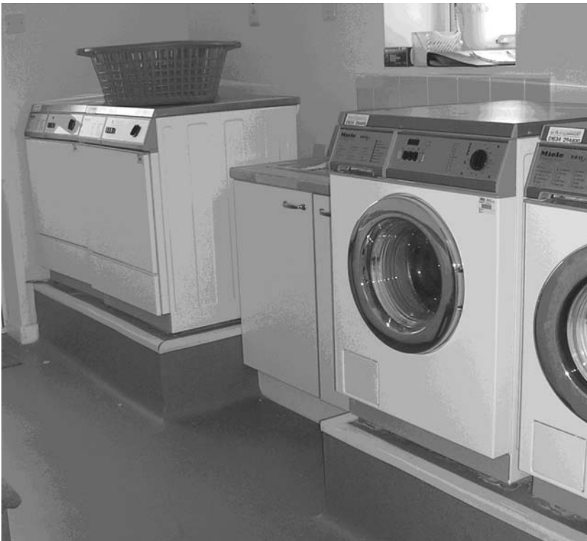
Figure 22.4. Laundry in the same building that has not benefited from a tenant-centred refurbishment
