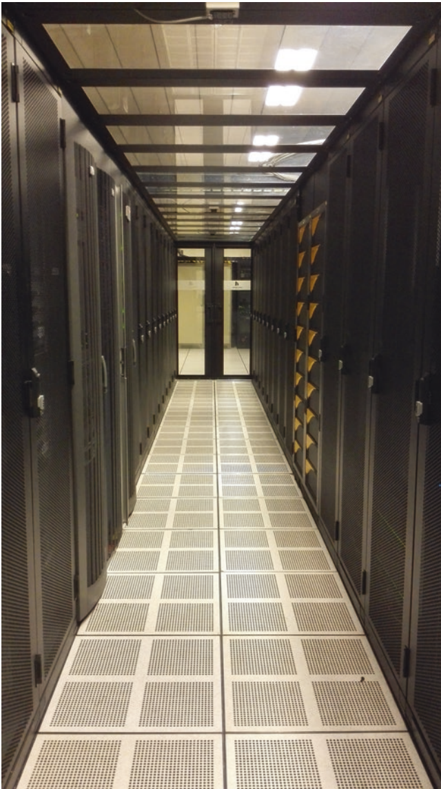
Fig. 17.4 This figure shows a server farm in a data center
