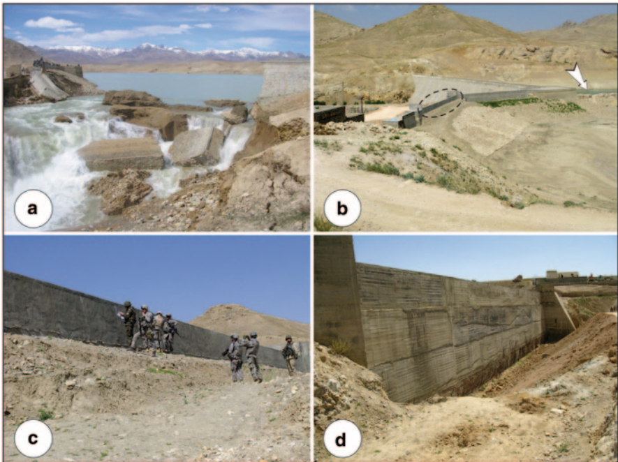
Fig. 4 Band-e Soltan dam; arrow in “b” is pointing to the original, tenth-century portion and dash-encircled section is the repaired wing-wall section represented in a, c and d. a March 2005 collapsed wing-wall section; b overview of the dam facing westerly; c author (second from left ) inspecting the repaired wing-wall section (reservoir side) and d downstream section of repaired wing-wall. (August 2009; Photographs by author)
