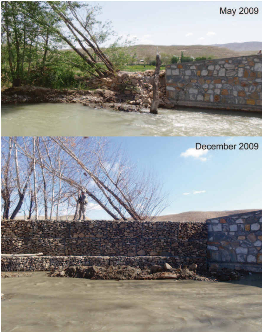
Fig. 6 Jungihal Bagh Demonstration Farm (Ghazni District) gabion-training/emplacment project photographs. Notice the sapped, dry-stacked rocks in the upper image, which did not minimize bank erosion behind the abutment. These rocks in the May 2009 image had been placed approximately 2 months prior to this picture being taken. After the training program, the section was protected with gabions ( lower image). (Photographs by author)
