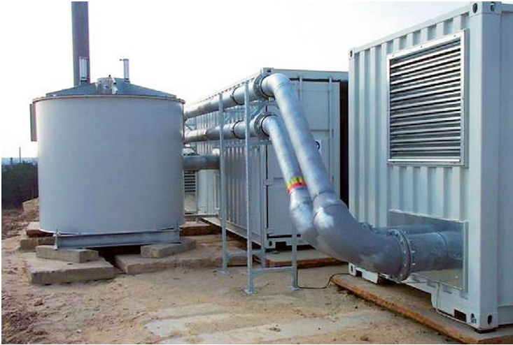
Fig. 14.14 Blower housing and exhaust gas treatment system at a closed landfill (Photo courtesy of Marco Ritzkowski)
