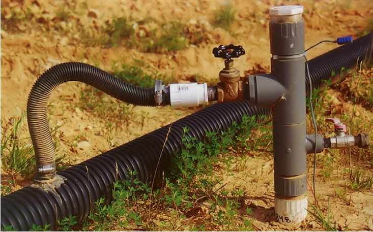
Fig. 14.18 Distribution manifold and air addition well for an aerobic landfill in the Southeast US
