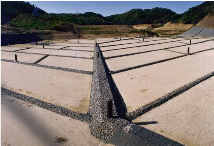
Fig. 14.10 LCRS of semi-aerobic landfill after construction and before waste placement; connected rock drains are shown (Photo courtesy of Yasushi Matsufuji)
