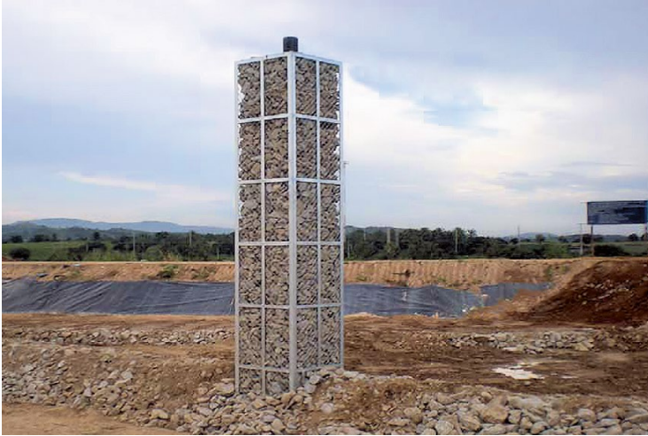
Fig. 14.12 Vertical vent of a semi aerobic landfill after construction and before waste filling
