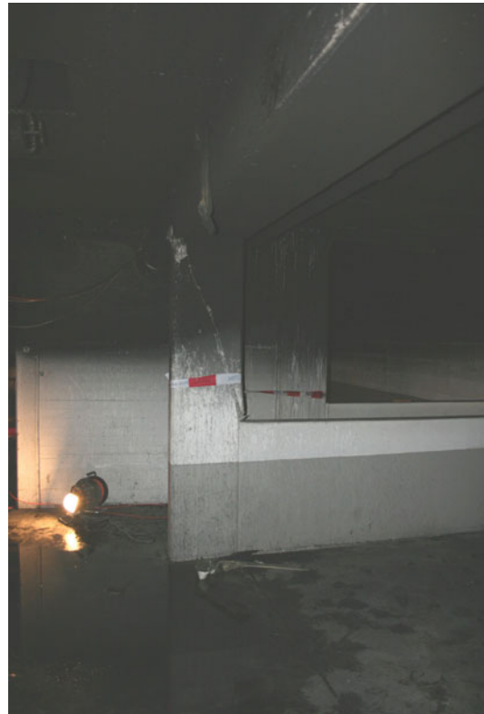
Fig. 52.7 Concrete columns that failed in shear due to thermal elongation of the ceiling
