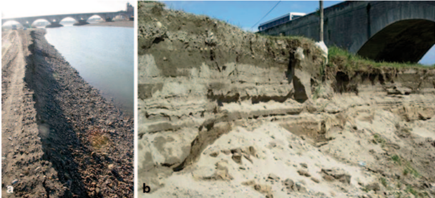
Fig. 13 Photographs of erosion of the left bank of the Rhône River upstream of Pont-Saint-Esprit bridge. Left photo : lateral erosion of a former gravel bar; right photo : lateral erosion of sandy top layer. In the back ground the mediaeval Pont-Saint-Esprit bridge. (Courtesy: NRC)
