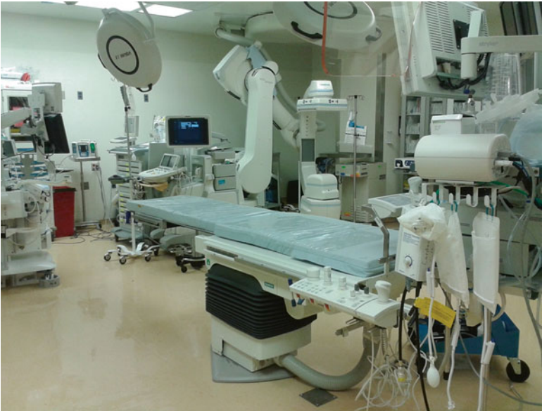
Fig. 19.8. Trauma hybrid operating room at RA Cowley Shock Trauma Center. Angiography capability is provided by Siemens Artis Zeego system whose C-arm is advanced into the operating field when needed and returns to its stored position away from the table during open procedures.
