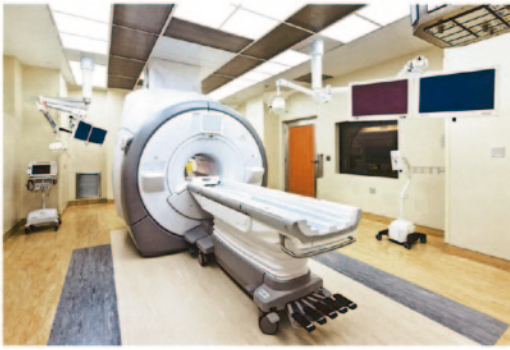
Fig. 1.1 3T magnetic resonance imaging (MRI) image-guided interventional OR. Diagnostic and interventional systems are integrated into standard OR environments with common controls and information displays. LED installation matches fluorescent lighting in adjacent ORs
