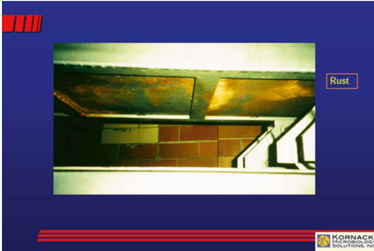
Fig. 7 Rusty underside of a catwalk for spray dryer
