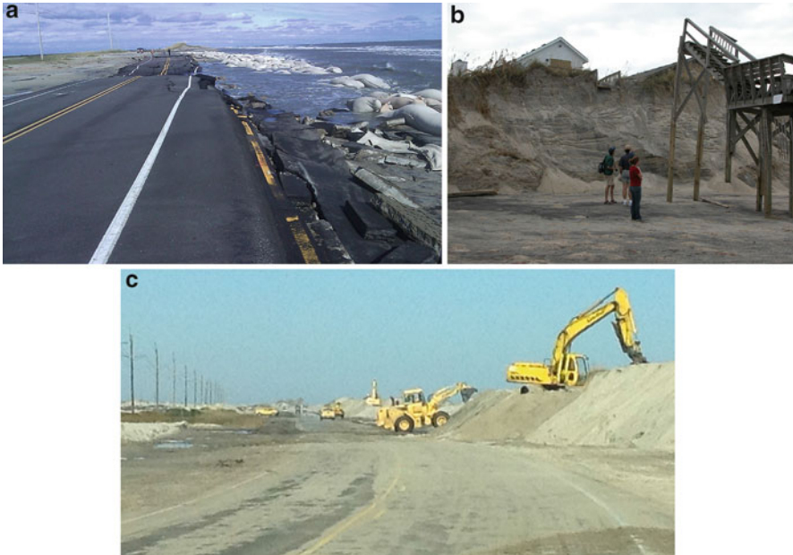
Fig. 1.1 Coastal management challenges on North Carolina Outer Banks: (a) storm impacts in Rodanthe (Hurricane Sandy, NCDOT 2012); (b) beach erosion in Nags Head (Hurricane Isabel, USGS 2003); (c) sand transport threatens homes and infrastructure (Nor'easter Athena, NCDOT 2012)
