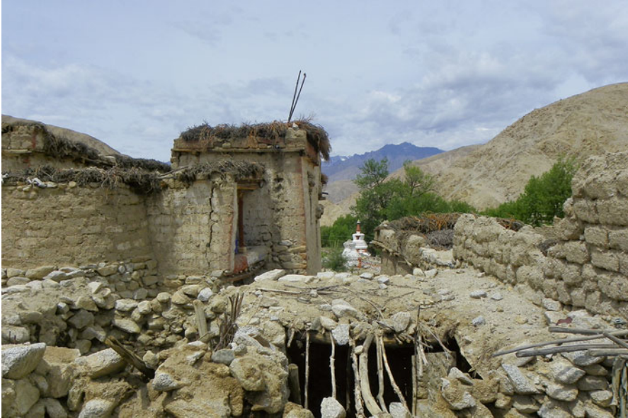
Fig. 5.5 Damage in the village of Igu Ladakh. Photograph J. Hurd
