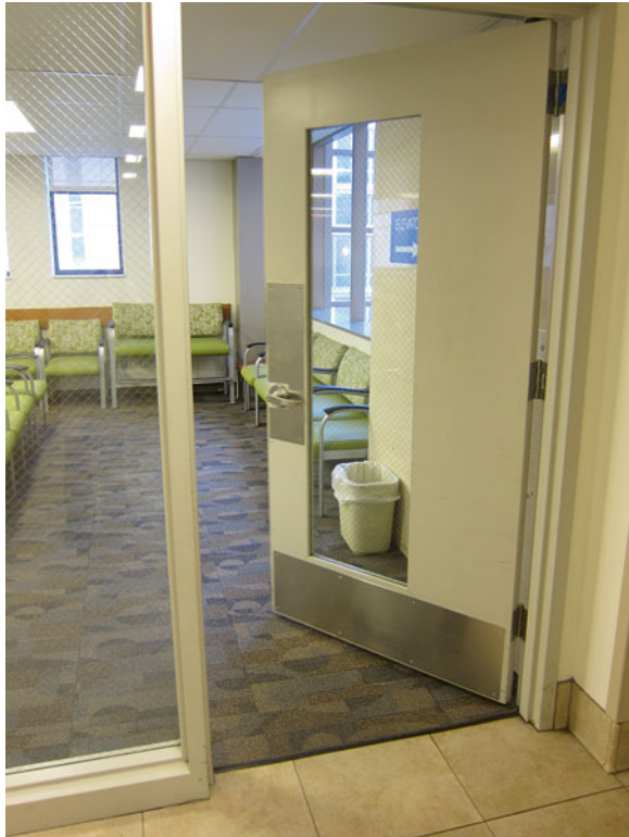
FIG. 4. Electronically powered and larger width doors as entryways either into a patient room in the hospital or in this case into the waiting area of the outpatient office are necessary.
