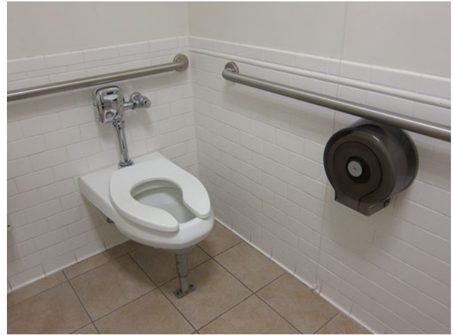
FIG. 5. Bathrooms should have floor mounted toilets with properly installed grab bars to prevent patient falls.
