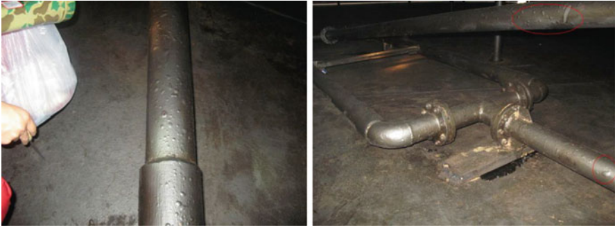
Fig. 4 The coating blister of the central drain pipe
