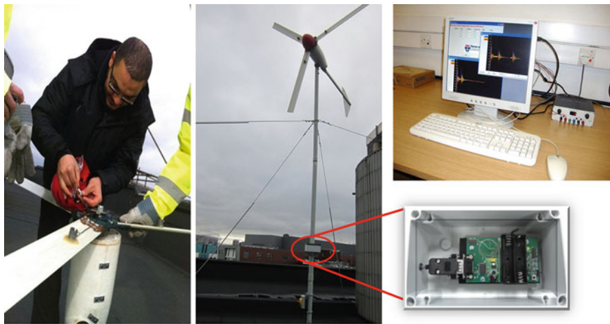
Fig. 2 System installation on the school's roof for field studies and the PC base station in the lab
