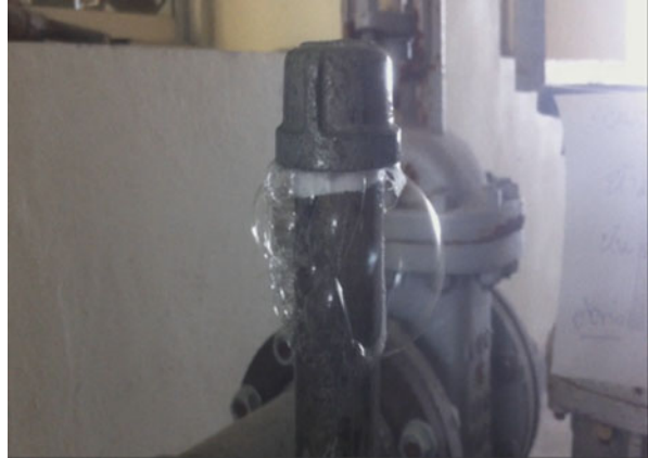
Fig. 2 Soap test on 20 ml/s leakage of pipe cap
