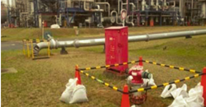
Fig. 1 Underground pipeline for fire extinguisher
