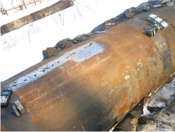
Fig. 6 A pipeline whose thickness was reduced up to 50 % of its original value aside of the segment between the sensors
