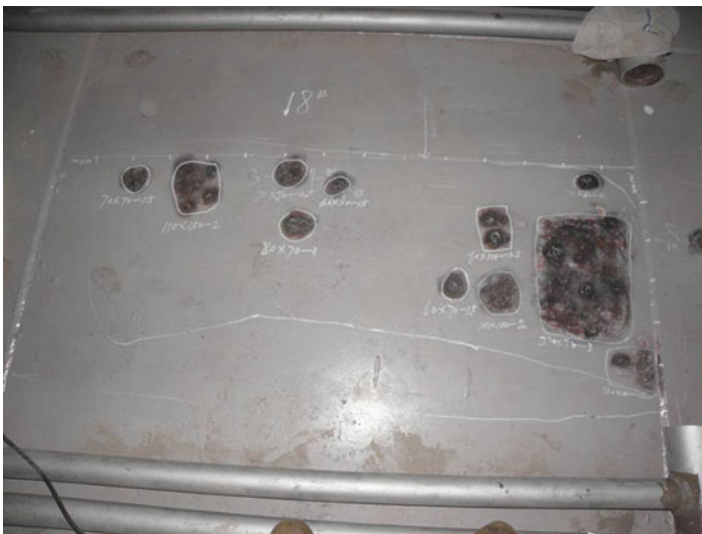
Fig. 5 Corrosion pits on the plate
