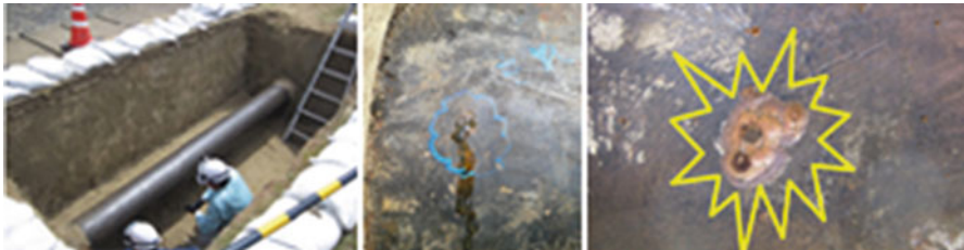
Fig. 6 Visual inspection of pipe defected at estimated area
