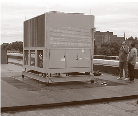
Fig. 11.67 An example of a rooftop chiller enclosure (courtesy of Acentech Inc., Cambridge MA)
