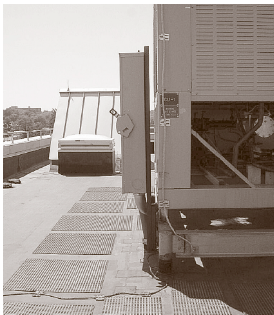
Fig. 11.65 An example of separating an electrical box from mechanical equipment to isolate vibrations
