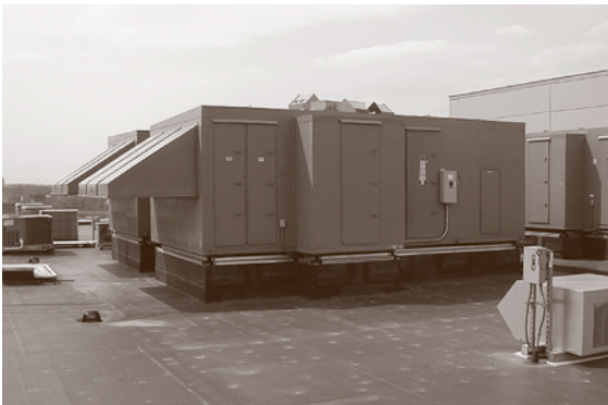
Fig. 11.66 An example of a rooftop HVAC unit enclosure (courtesy of Acentech Inc., Cambridge MA)
