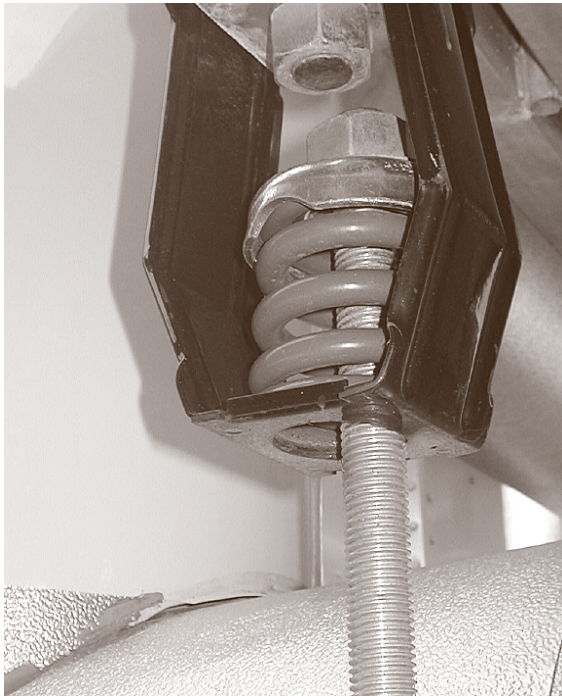
Fig. 11.56 A misaligned isolating pipe hanger. Note that the post is touching the support, thus short-circuiting the isolating effect of the hanger
