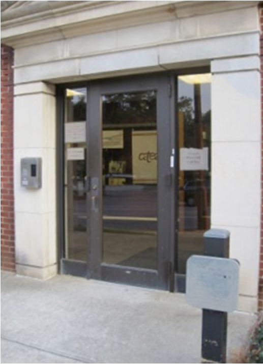
Fig. 23.8 Automatic motion sensor door opener. For buildings that have controlled access, keycards with embedded RFID tags permit hands-free access if the reader is located in the path of travel and at a height that is convenient for all employees
