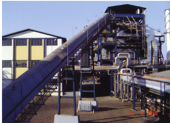
Fig. 3.5 High-pressure boilers at the Santa Adélia sugar mill in the state of São Paulo. (Photo courtesy of CENBIO)
