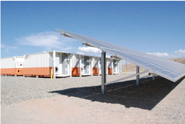
Fig. 9 Prosperity solar energy storage project, New Mexico featuring both voltage smoothing and peak shifting
