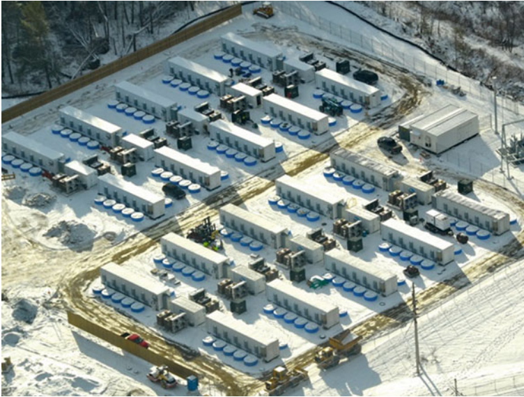
Fig. 8 Beaconpower 20 MW/5 MWh(15 min storage) flywheel demonstration in New York State
