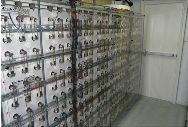
Fig. 11 UltraBattery cell bank at Hampton Wind Farm
