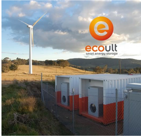
Fig. 10 1 MW UltraBattery storage system at Hampton Wind Farm
