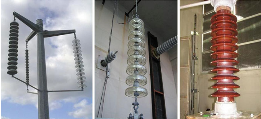
Fig. 11 View of high voltage insulators for salt deposit measurements and for laboratory tests
