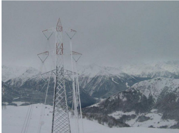
Fig. 12 Wet-snow accretion on overhead line during a heavy snowfall in the Alps
