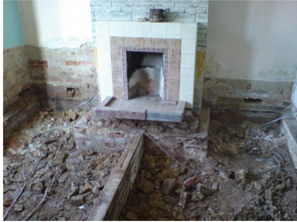
Fig. 9.2 The late nineteenth-century soil foundation of my family home, an act of excavation through rotten floorboards which exposed a network of cables. (Photograph by Christine Finn)
