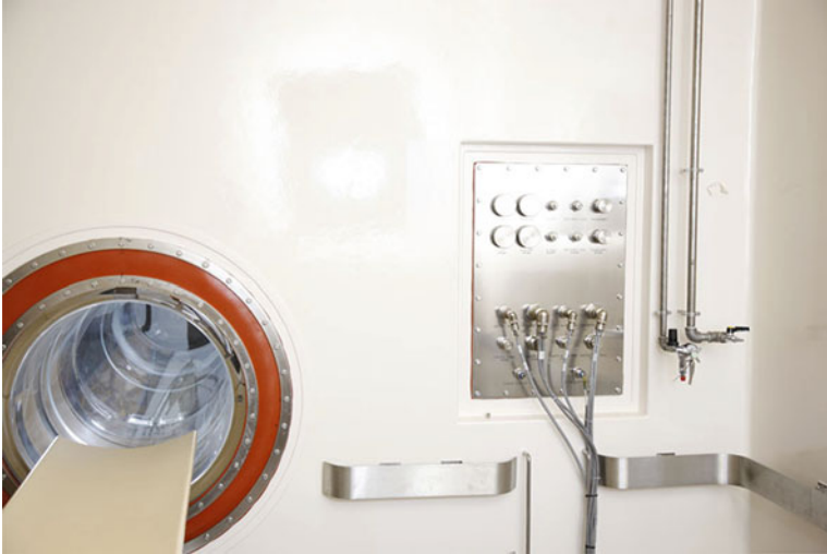
Fig. 10.2 Airtight patch panel through which electrical signals are sent to electronic components on the cold side of the barrier wall. This eliminates the need for electronic components to be on the hot side and subjected to decontamination chemicals
