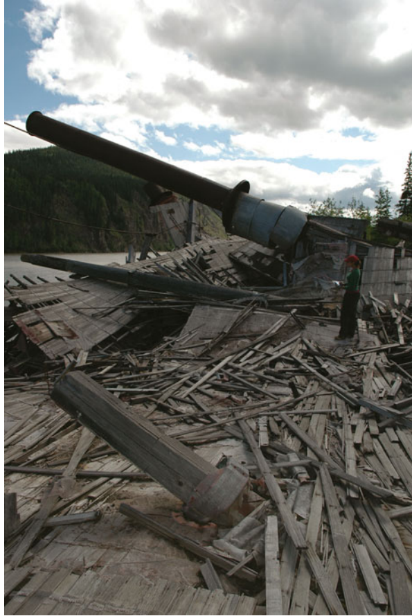
Fig. 9.4 The collapsed superstructure of Seattle No. 3 in 2010. (Photograph by John Pollack 2010)
