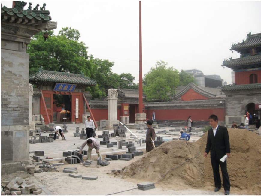
Fig. 10.5 Making Dongyue temple more accessible in 2008 meant renovating the entrance and adding wheelchair ramps. (Photo by author)
