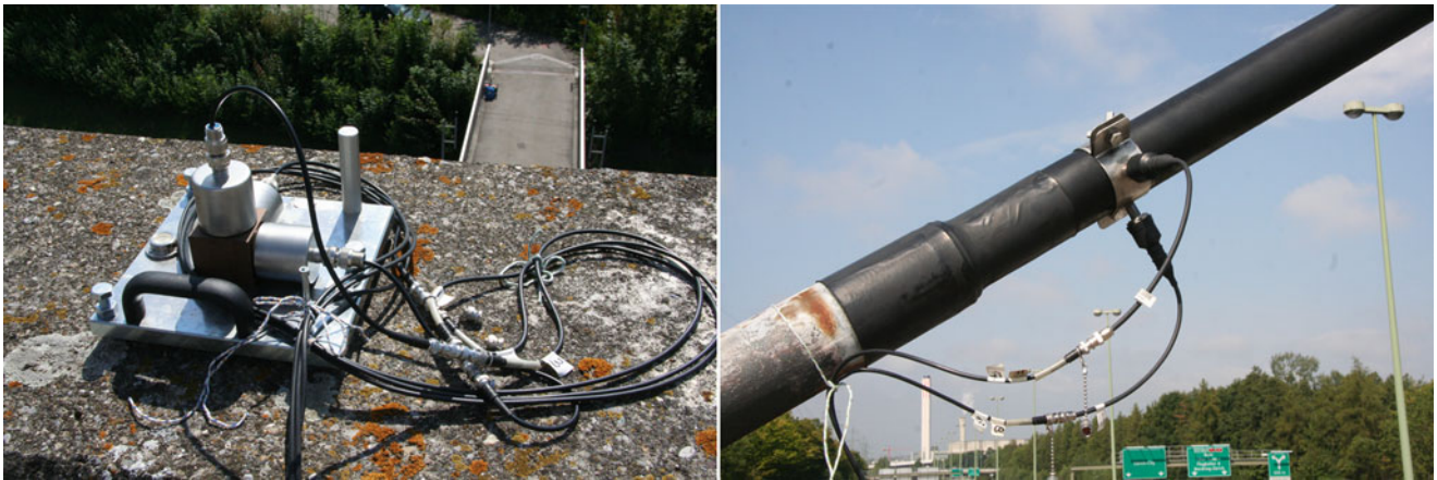
Fig. 2.10 Sensors at the pylon tip ( left ) and at a cable ( right )
