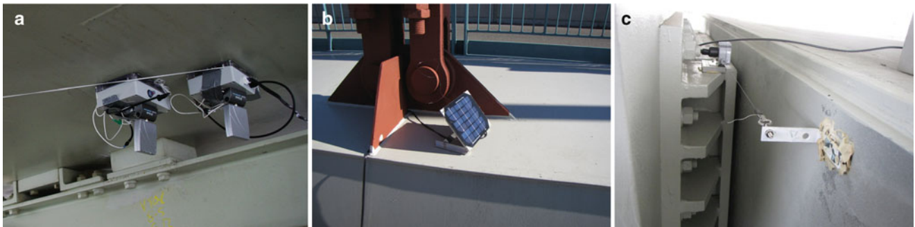
Fig. 8.2 Installation details of the New Carquinez Suspension Bridge long-term monitoring system: (a) typical Narada wireless sensor node beneath the deck girder in a magnetically mounted weather-proof enclosure; (b) small solar panel installed on the bridge top deck to power a Narada node; (c) string potentiometer at the deck-tower interface to measure longitudinal displacement
