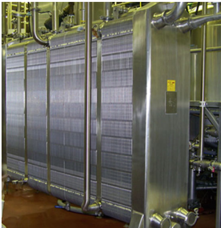
Fig. 5.5 A plate heat exchanger used for cooling of mixes following batch pasteurization. This also provides a good illustration of plate heat exchangers used for HTST pasteurization, when properly configured
