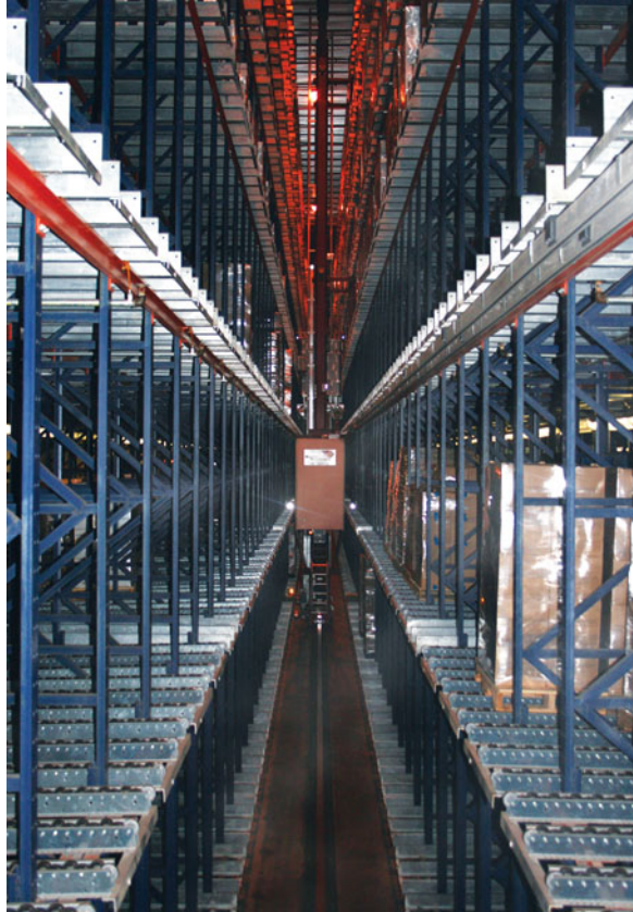
Fig. 10.12 Multiple story storage/retrieval system capable of moving product into and out of storage by computer-controlled vehicles (courtesy of Westphalia Technologies, Inc., York, PA)
