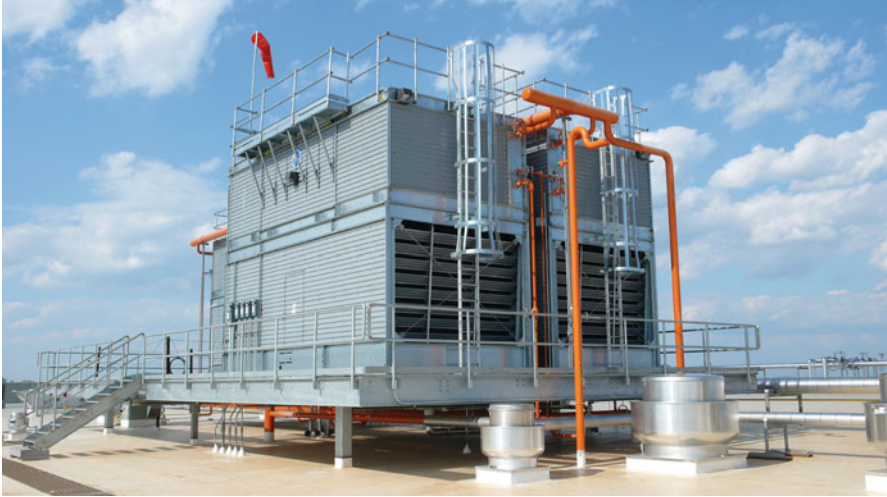
Fig. 7.28 Field installation of an evaporative condenser on an industrial ammonia refrigeration system (courtesy of Baltimore Air Coil, Jessup, MD)
