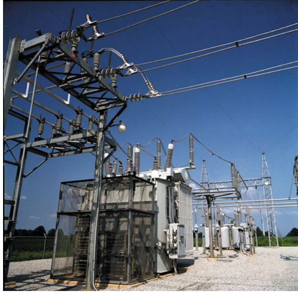
Fig. 2.33 Distribution substation view (Courtesy of General Electric)
