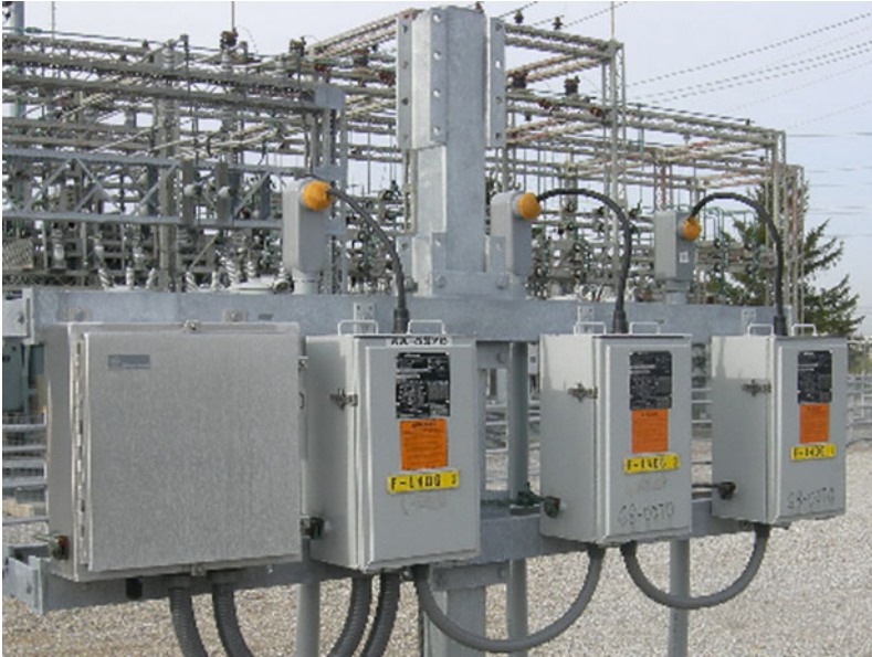
Fig. 2.20 Three-phase station voltage regulator
