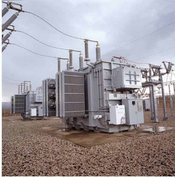
Fig. 2.26 Voltage transformers (Courtesy of General Electric)
