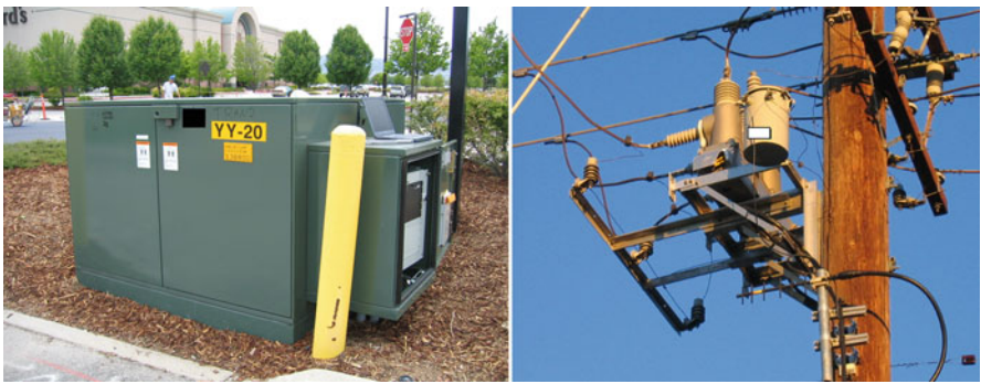
Fig. 2.7 Typical pad-mount and pole-mount switches
