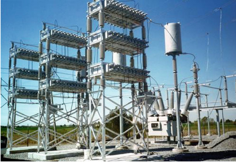
Fig. 2.31 Capacitor Bank (Courtesy of General Electric)
