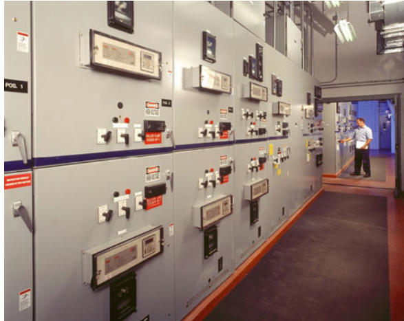
Fig. 2.28 Indoor switchgear front view (Courtesy of General Electric)
