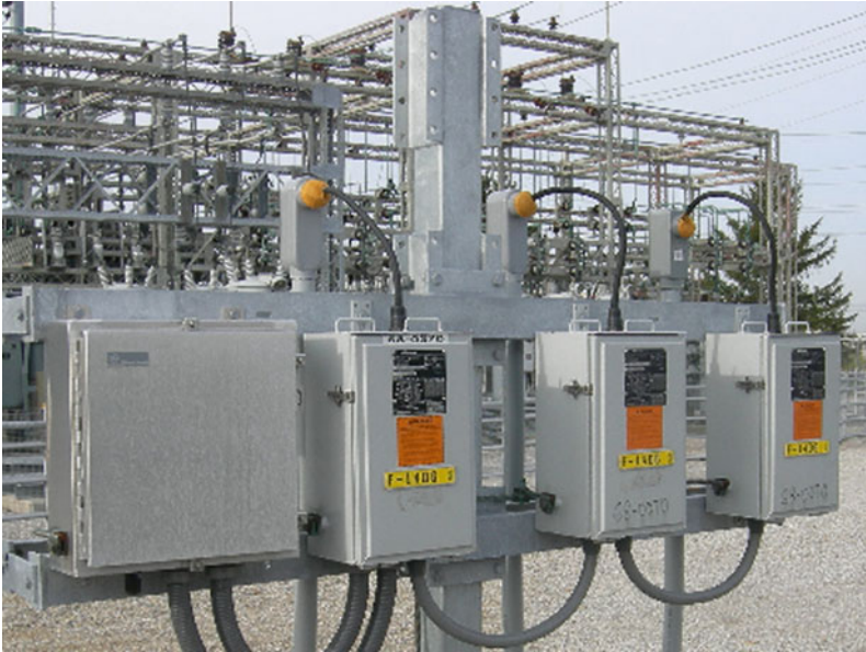
Fig. 2.20 Three-phase station voltage regulator
