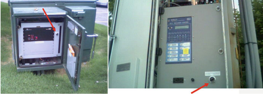
Fig. 2.6 Pad-mount controller and pole-mount reclosing relay with enable/disable switches
