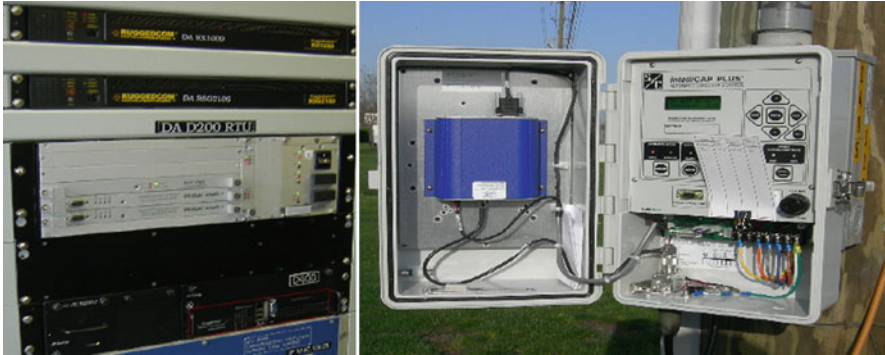
Fig. 2.19 Example station and feeder voltage/VAR control devices
