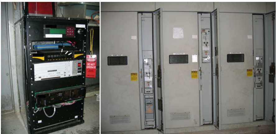
Fig. 2.8 Typical substation controller and vault switch
