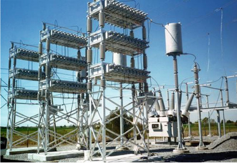
Fig. 2.31 Capacitor Bank (Courtesy of General Electric)
