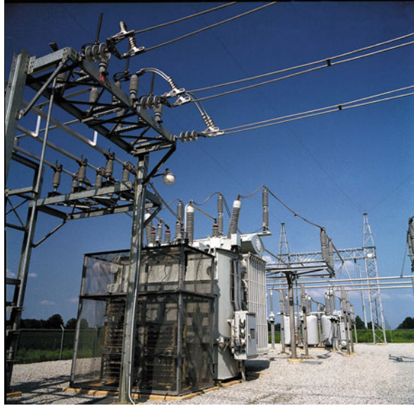
Fig. 2.33 Distribution substation view (Courtesy of General Electric)
