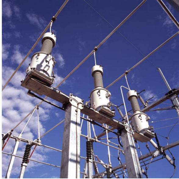
Fig. 2.27 Outdoor switchgear busbar (upper conductors) with voltage transformers (Courtesy of General Electric)
