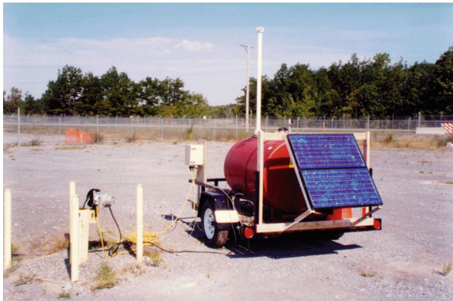
Fig. 13.2 Example of solar powered system with photovoltaic panels for powering product skimming
